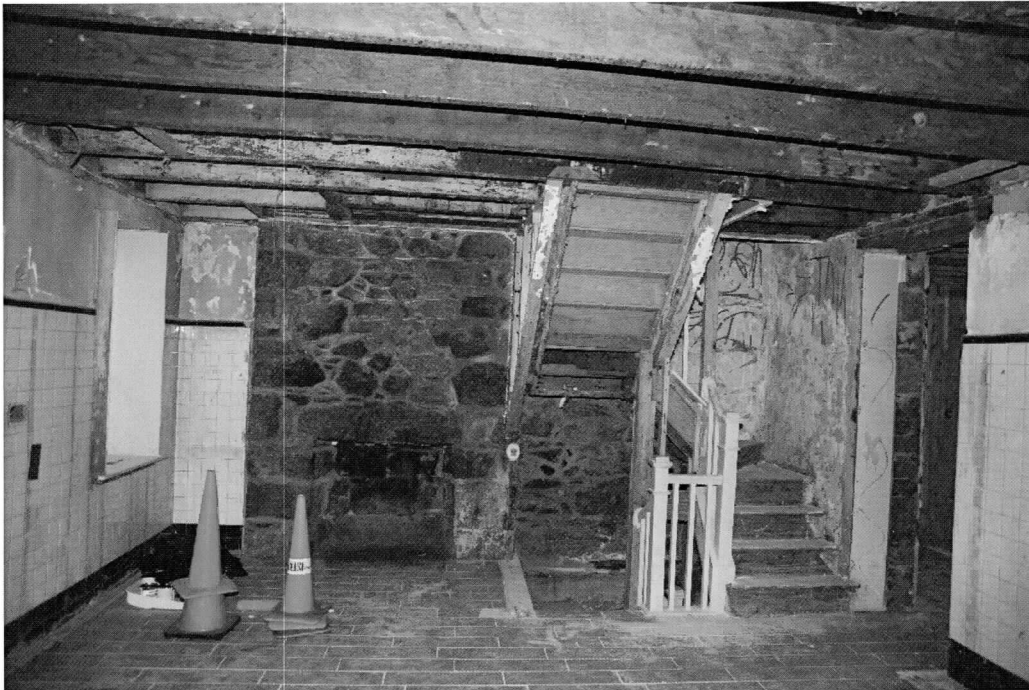
Photo 7 of 18: First story east wall after removal of most later additions, with rebuilt stair. 11/5/2019
