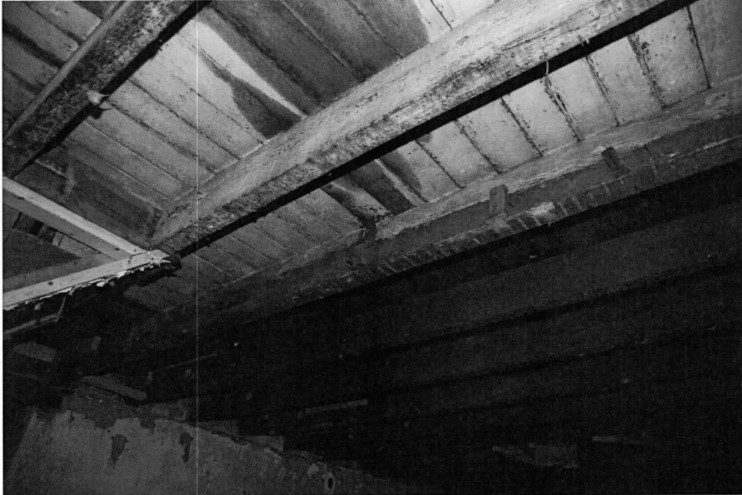
Photo 9 of 18: First story ceiling framing showing evidence of missing partition wall. 11/5/2019
